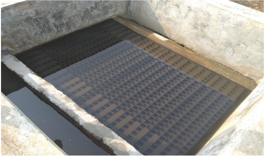
Tube settler clarifier
