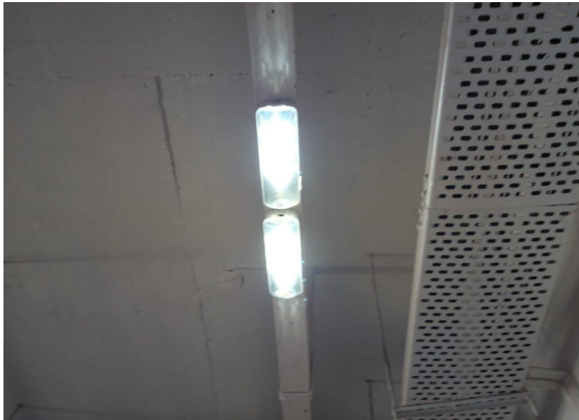
Mechanical ground floor LED
