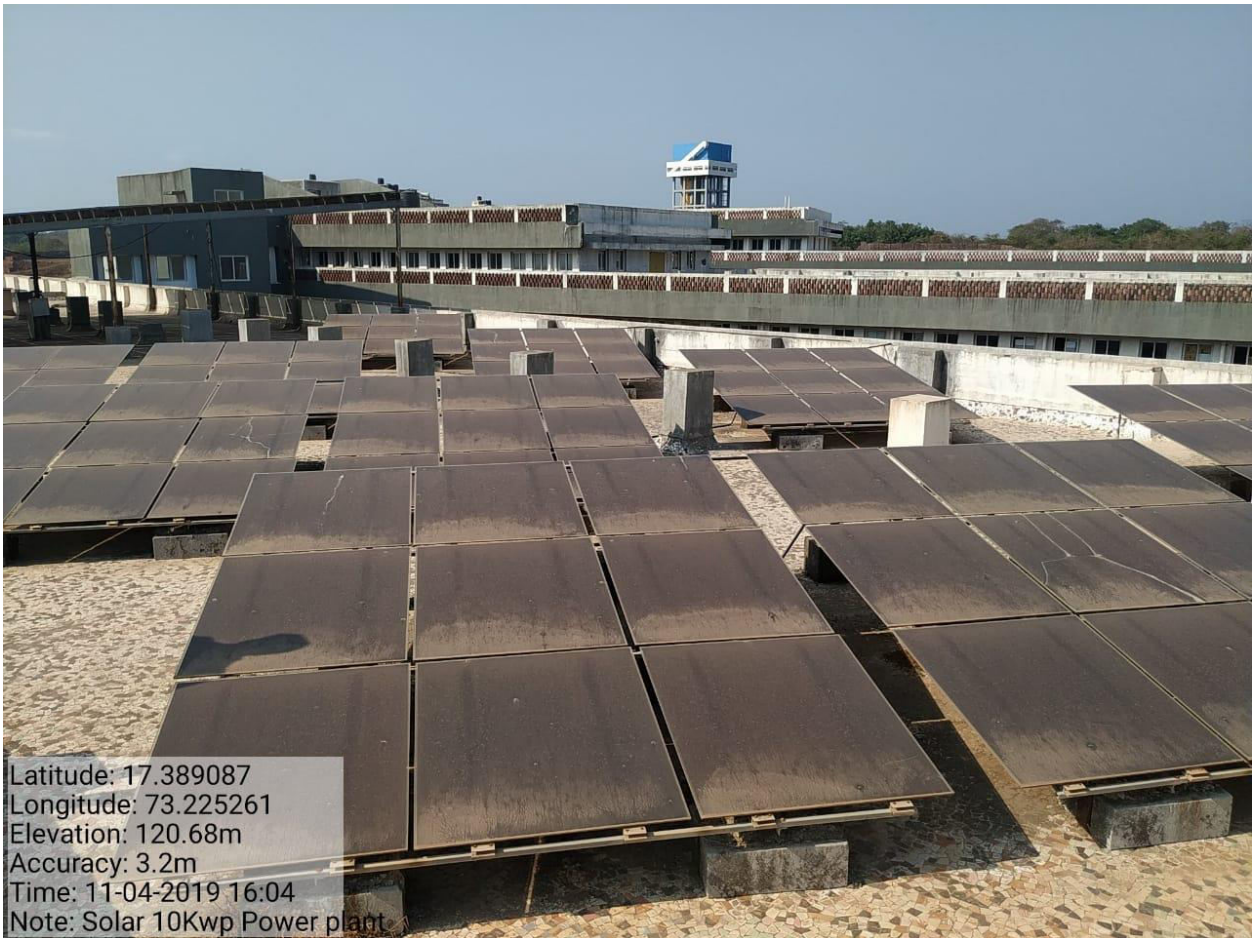
Solar on Sripati A1 Building
