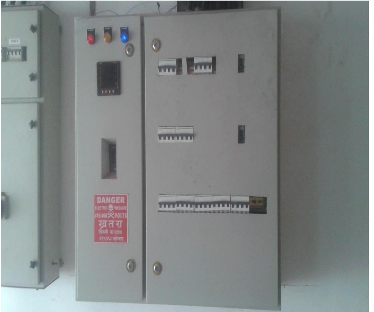
Incoming feeder of solar.
